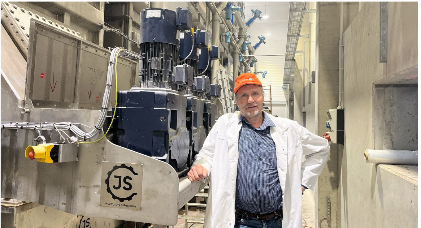
Markus Beckmann, Bioceval GmbH & Co. KG, at the completed raw material intake facility. (Photo:
